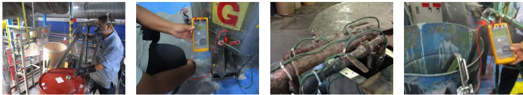
Improvements of grounding-bonding system improvements and availability checks to prevent fire risks
